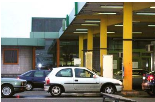
Fig. 7: Installation of fix-installed monitors at the car lane at the ITRAP field test site Nickelsdorf.
